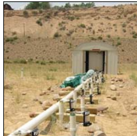
Wells at old Rifle mine inject acetate (vinegar) into the ground to stimulate the growth of microbes already in the soil.
